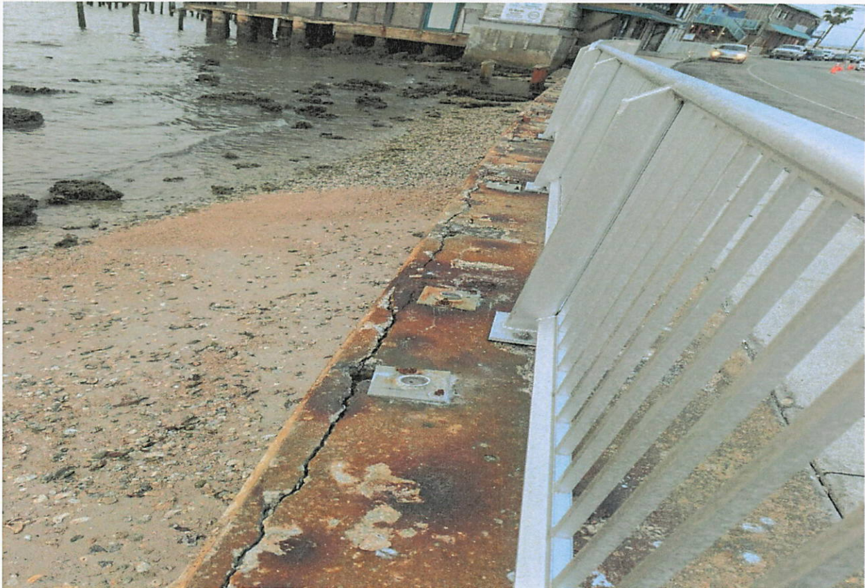
Existing Seawall Exhibiting Delamination
