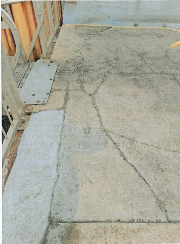
Typical Sidewalk Cracking
