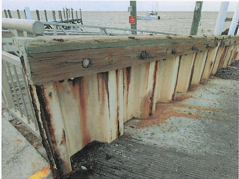
Existing Ramp Coating Damage
