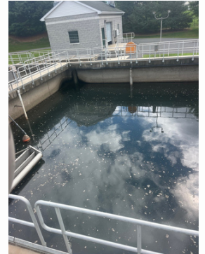
South Plant in anaerobic stage
