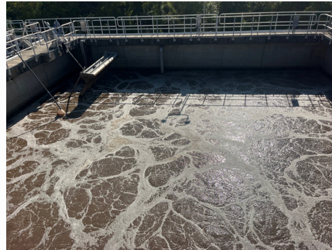
North Plant tank aerobic stage
