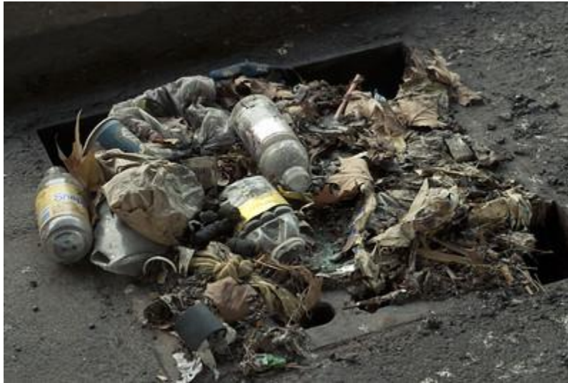
Clogged storm drain. (Photo by Chris Hamby licensed as CC BY-SA)
