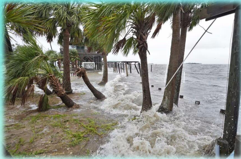
Hurricane Debby (August 5, 2024). Surge, wind, and flooding caused additional damage to structures and infrastructure already weakened by Idalia.
